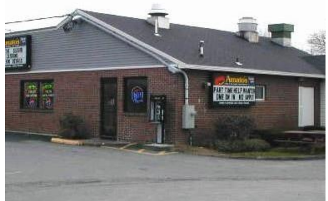
HVAC equipment and service connections are highly visible, adding unnecessary clutter to this small restaurant.
